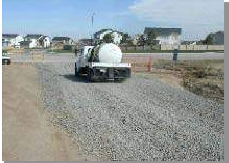
Photograph DC-1. Water truck used for dust suppression. Photo courtesy of Douglas County.
