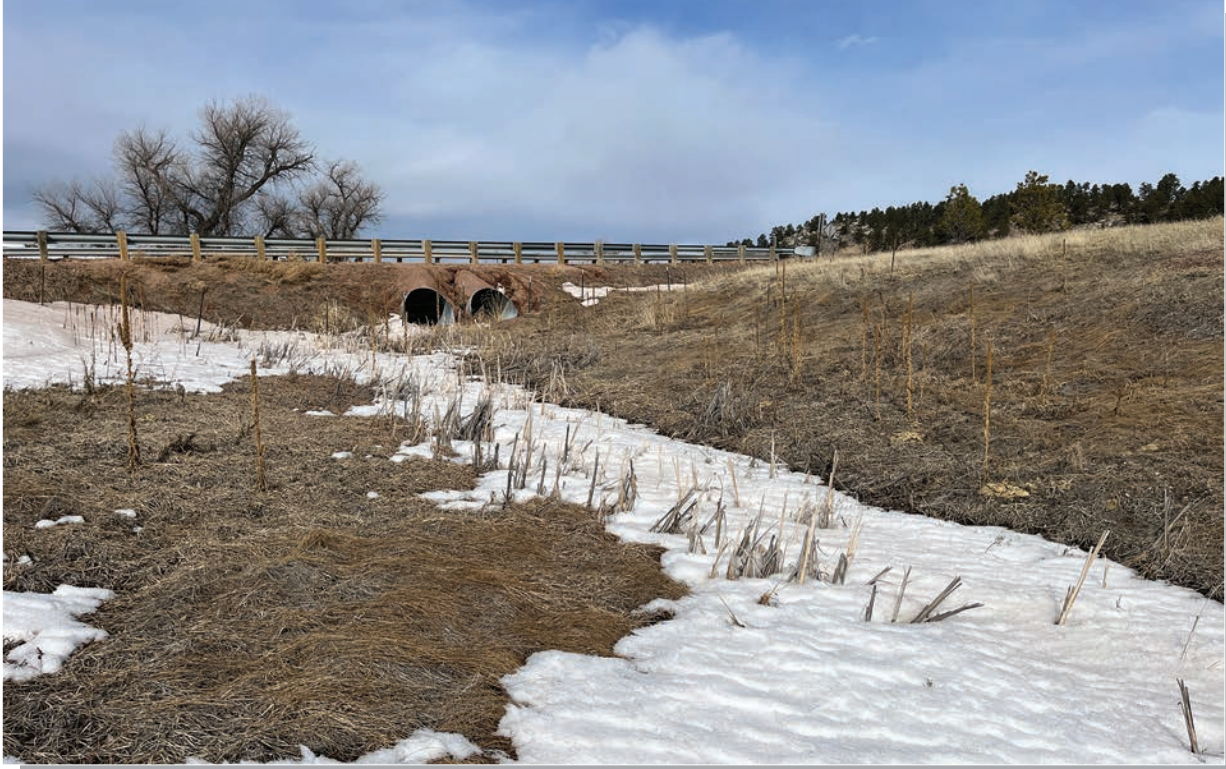
Photo 7 - Another section of drainage 1 in the project area. View is to the northwest.
