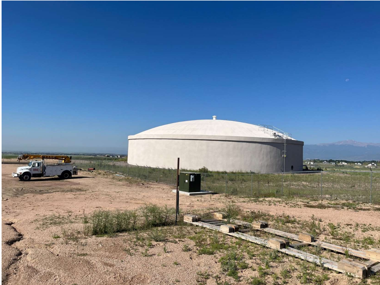
PHOTO 2 – View of the water tanks located at the northernmost edge of the site, facing southeast. Flora and fauna are sparse in the areas where construction vehicles and materials are stored, and construction activities are ongoing. Some noxious weeds are present near this area.
