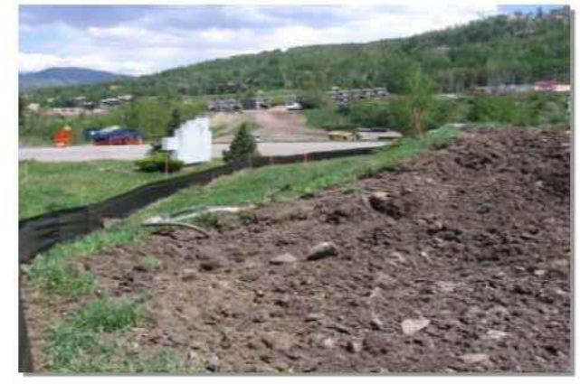
Photograph SP-1. A topsoil stockpile that has been partially revegetated and is protected by silt fence perimeter control.
