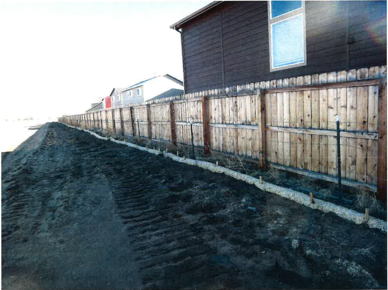
Photo #3 - Straw barrier on east boundary of Bent Grass Filing #2 adjacent to west boundary of Phase 1 Challenger Homes (view looking north)
