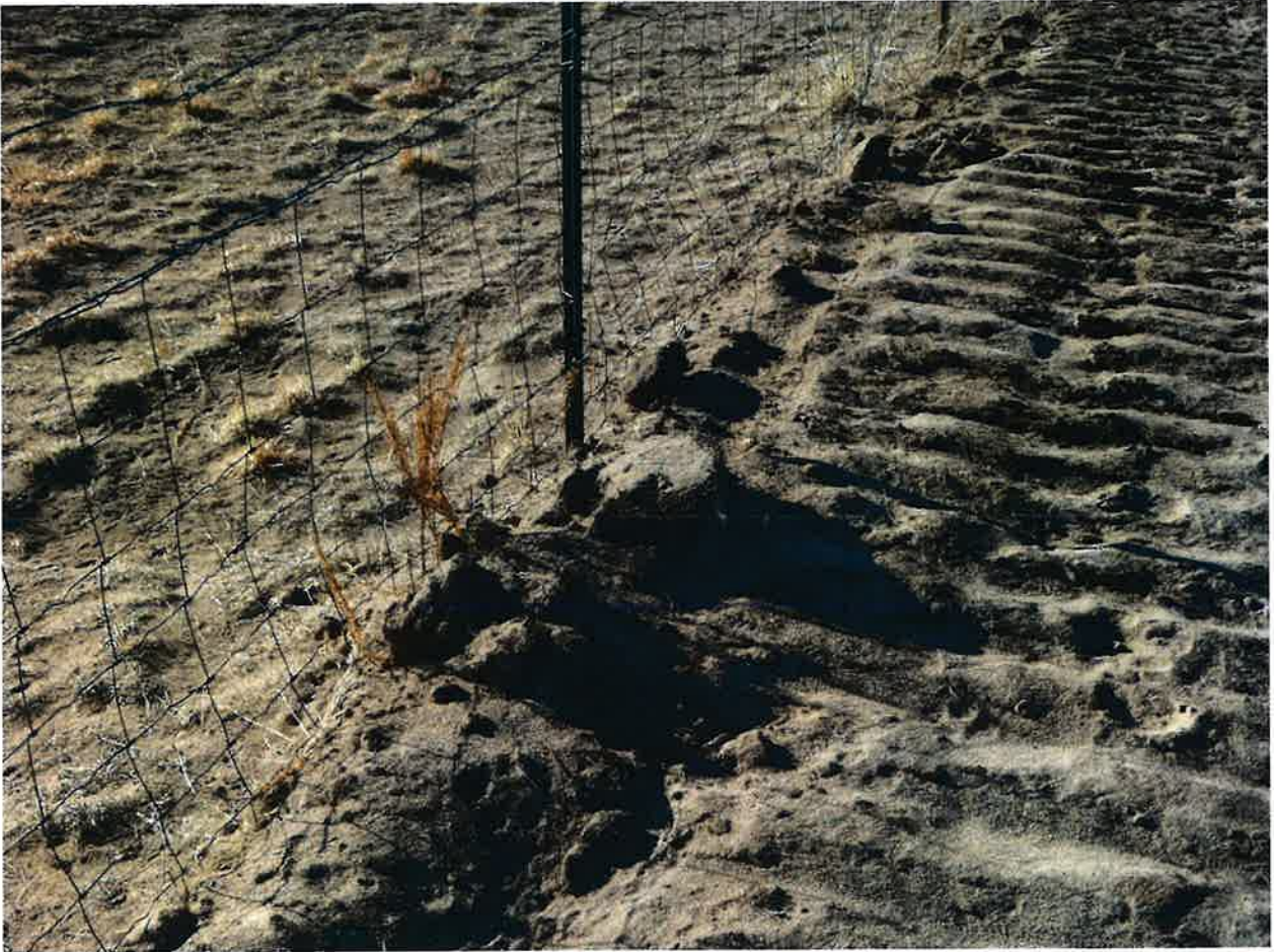
Photo #2 - Closeup of graded dirt forcing our fence out of position and encroaching on our property
