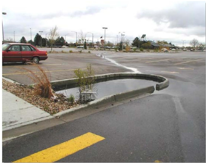
Photograph B-4. Runoff passed the upgradient rain garden, shown in Photo B-3, and flooded this downstream rain garden.
