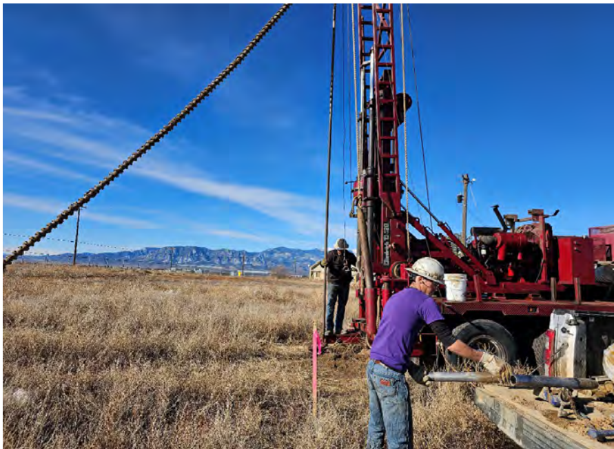
Photo No. 6 Location: Boring B-1 Date: 02/14/2024 Two truck mounted drill rigs equipped with solid stem augers were used for drilling. Samples were collected utilizing California barrel samplers.
