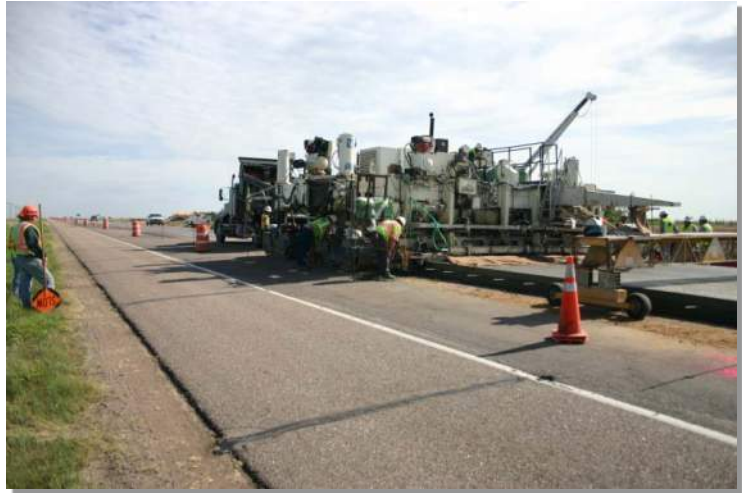
Photograph PGO-1. Paving operations on a Colorado highway. Photo courtesy of CDOT.
