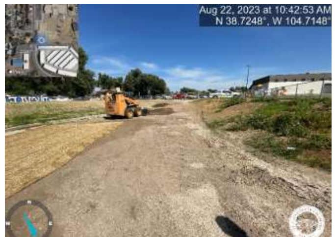
Photo 12: Remove excess sediment from the maintenance access road and reestablish road base.
