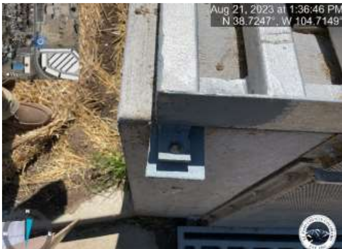
Photo 3: Pond: Install bolts or locks on grate per the approved plans. Reference sheet C8.1 of the Construction Documents.
