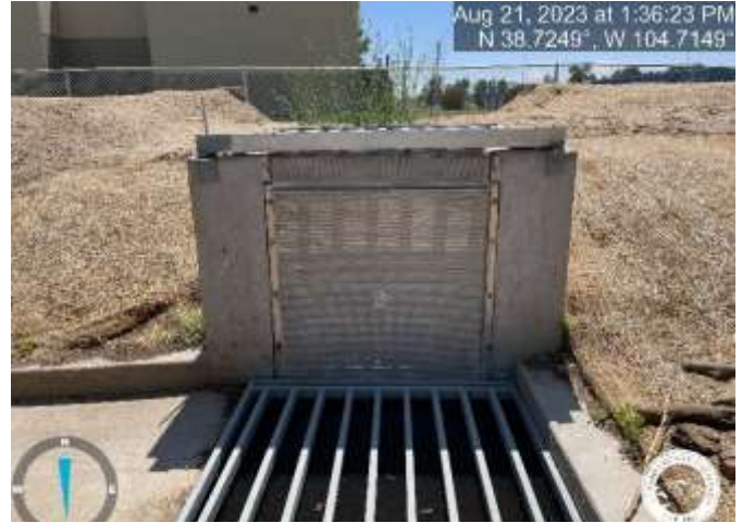
Photo 2: Pond: Replace trash screen with No. 93 Johnson Vee Wire or Equivalent. Reference sheet C8.1 of the Construction Documents.
