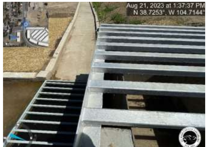
Photo 4: Pond: Install concrete cross-member or equivalent between the trash screen and orifice plate gap. Documents. Reference sheet C8.1 of the Construction Documents.
