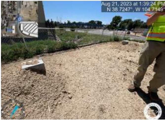
Photo 5: Confirm installation of the emergency overflow spillway. Spillway should be trapezoidal, 5' Weir width, with 4:1 slopes of 4' on either side. Reference sheet C8.1 of the Construction Documents.
