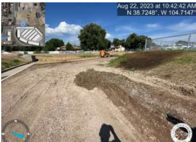
Photo 11: Remove excess sediment from the maintenance access road and reestablish road base.
