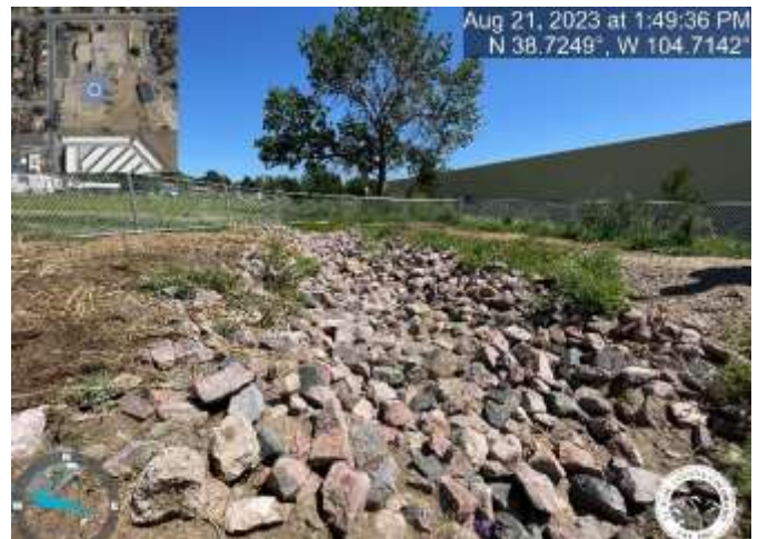
Photo 8: Riprap rundown is not 43.77' in length. Extend riprap to, at a minimum, the fence line and reflect change on as-builts
