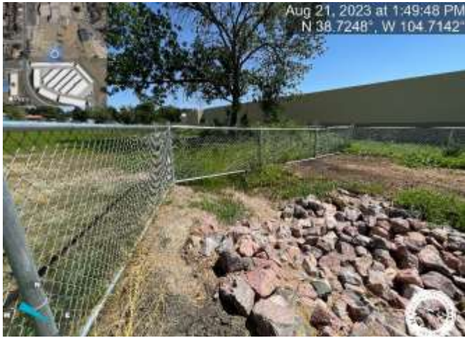
Photo 9: Riprap rundown is not 43.77' in length. Extend riprap to, at a minimum, the fence line and reflect change on as-builts
