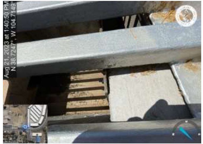
Photo 6: Confirm installation of gasket or silicone caulk around the orifice plate.
