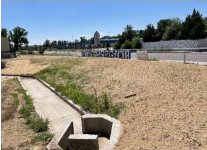
Photo 1: Pond: Install erosion control blankets along pond slopes per the approved Grading and Erosion Control Plan and notes.
