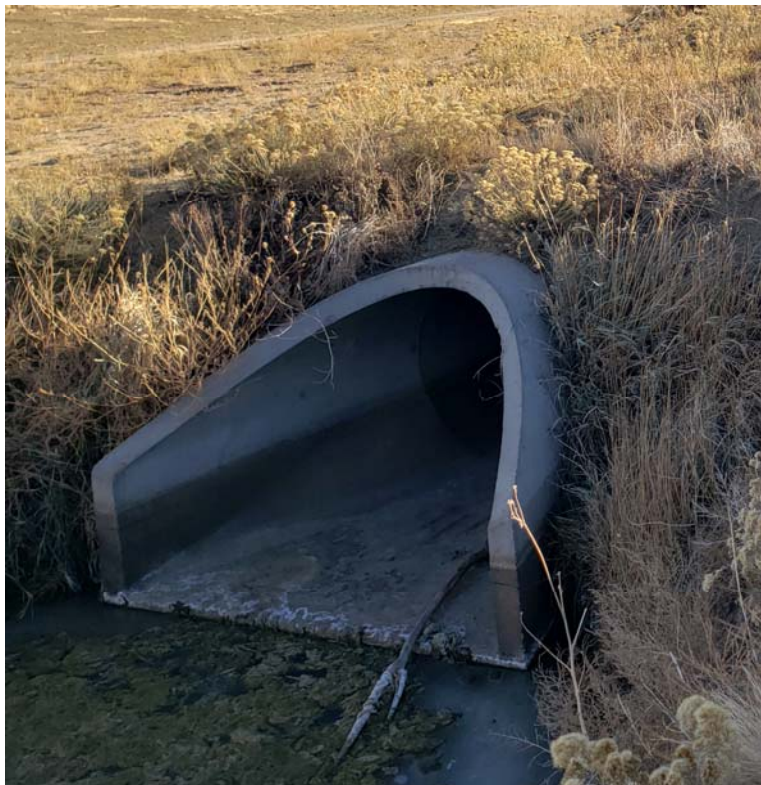
Figure 6-Existing 60" RCP FMIC Culvert in Glens at Widefield Filing No. 6 (South of Corvallis)
