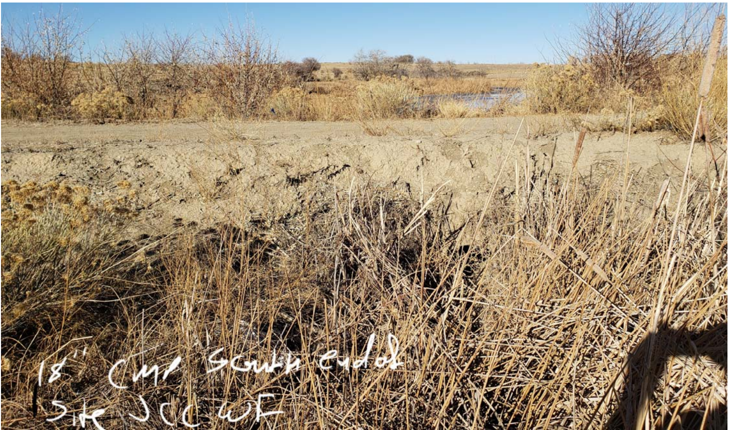
Figure 7-Existing 18" CMP and Embankment (Jimmy Camp Creek-West Fork) Located south of proposed Corvallis Development
