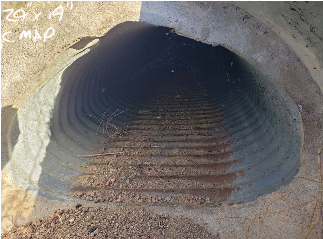
Figure 5-Existing 29" x 19" CMAP Fontaine Road Ditch Across Rolling View Drive (Appears to be grouted in insert) (NW of development)
