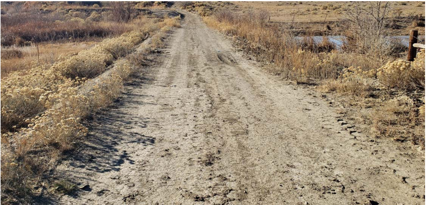
Figure 8-Existing 18" CMP and Embankment (Jimmy Camp Creek-West Fork) Located south of proposed Corvallis Development
