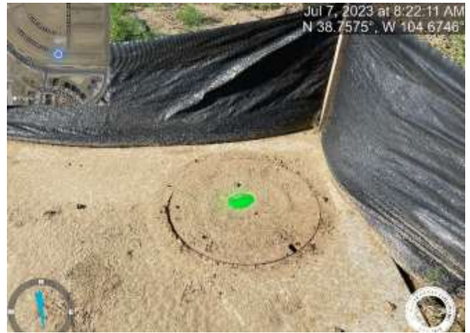
Photo 2: Example of marked stormwater inlet structure that needs to be cleaned of sediment and debris.
