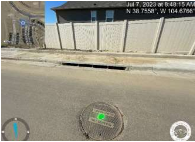
Photo 5: Example of marked stormwater drain structure that needs to be cleaned of sediment and debris. Not all marked inlets are depicted in these photos.
