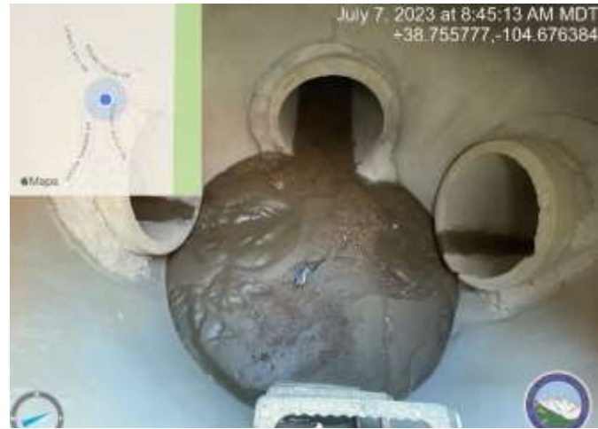
Photo 1: Example of storm drain that needs to be cleaned of sediment.
