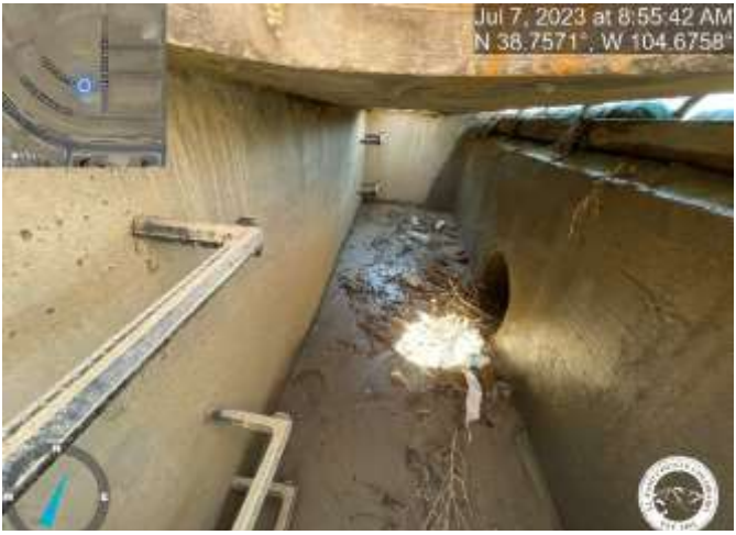
Photo 6: Example of stormwater inlet structure that needs to be cleaned of sediment and debris.
