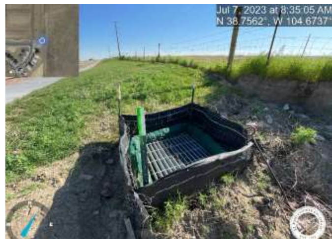
Photo 3: Example of marked stormwater area drain structure that needs to be cleaned of sediment and debris. Not all marked inlets are depicted in these photos.
