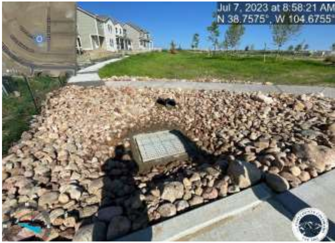
Photo 7: Example of marked stormwater area drain structure and culverts that need to be cleaned of sediment and debris.
