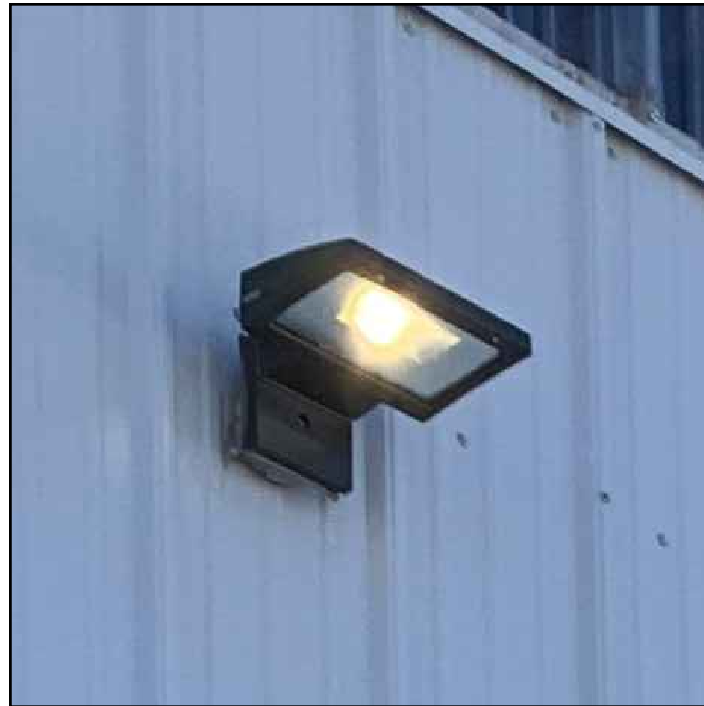
Wall Mounted Lighting
