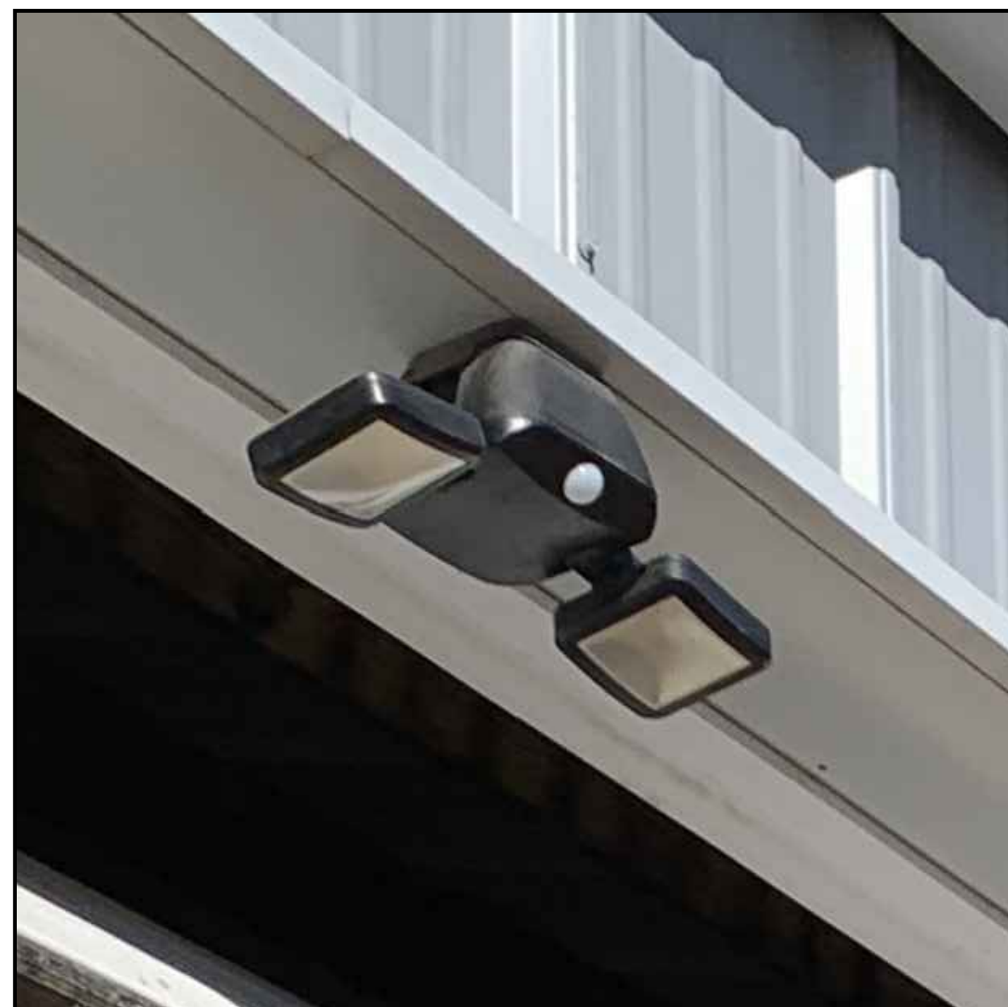
Wall Mounted Lighting
