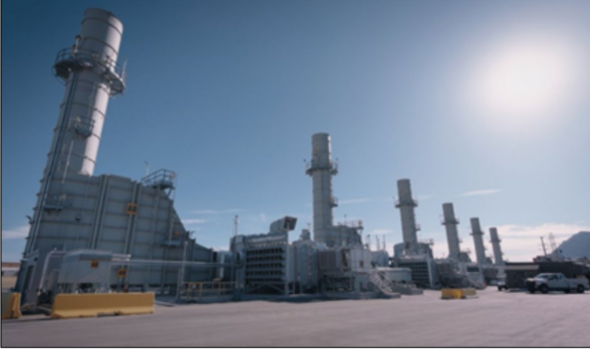
Figure A- 3: South Plant Aeroderivative Generators
