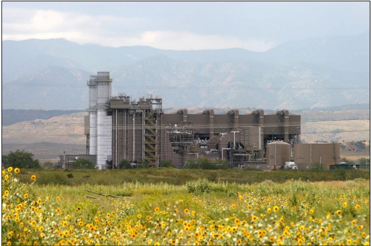
Figure A- 2: Front Range Power Plant
