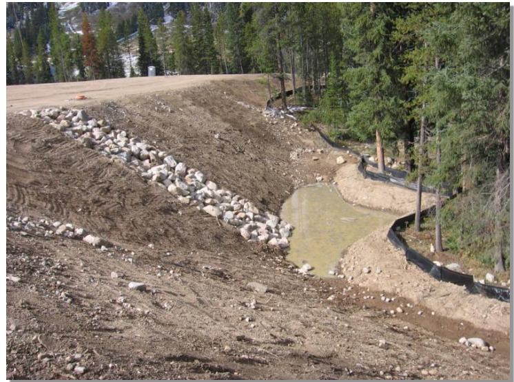
Photograph SB-1. Sediment basin at the toe of a slope. Photo courtesy of WWE.
