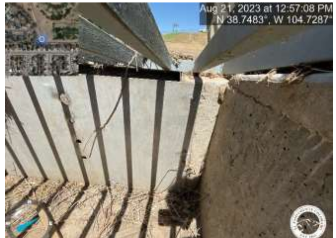
Photo 16: Pond: Confirm installation of gasket or silicone caulk around the orifice plate.
