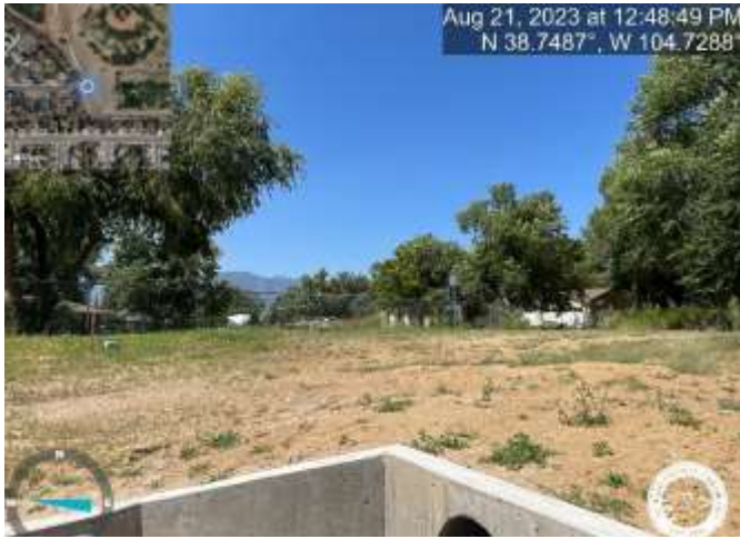
Photo 9: Pond: Confirm installation of the emergency overflow spillway. Spillway should be trapezoidal, 21' Weir width, with 4:1 slopes of 6' on either side. Reference sheet C7.5 of the Construction Documents.
