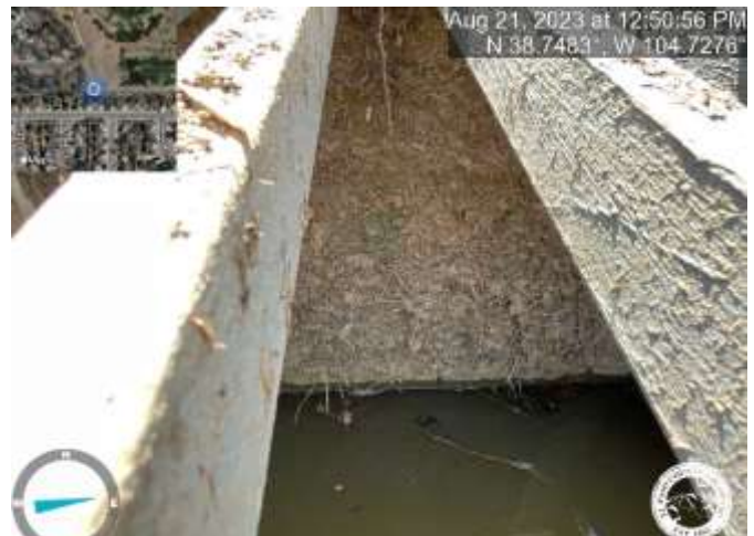
Photo 12: Pond: Replace trash screen with No. 93 Johnson Vee Wire or Equivalent. Reference sheet C7.5 of the Construction Documents.
