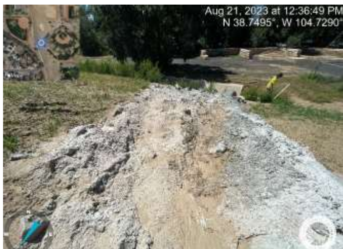
Photo 3: South of building: Remove and replace grouted riprap with 18" Type M riprap pad per the approved plans and for positive drainage and erosion prevention. The riprap needs to be shaped for positive drainage, currently the grouted riprap does not have a consistent shape with grouted rocks raised in the middle of the rundown. The riprap also should be buried in the ground so that the riprap is flush with the ground. Currently the riprap is a foot above the ground which is contributing to erosion from splashover especially downstream where the rundown meets the concrete lined channel. Reference sheet C8.2 of the Grading and Erosion Control Plans.
