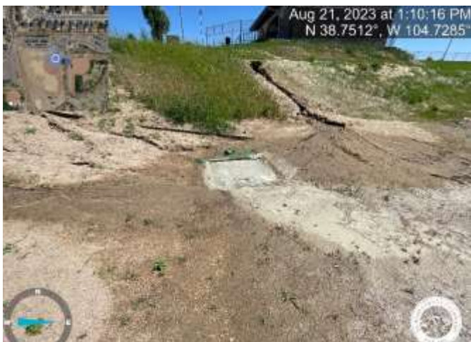
Photo 19: NE corner of building: Remove sediment/debris that is clogging the area drain.
