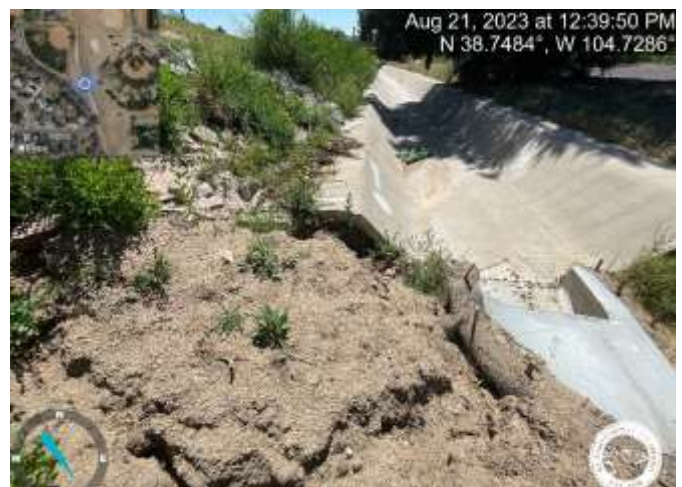
Photo 4: Repair riling below the grouted riprap to prevent erosion underneath the concrete channel.
