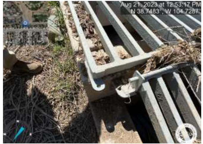
Photo 14: Pond: Install bolts or locks on grate per the approved plans. Reference sheet C7.5 of the Construction Documents.
