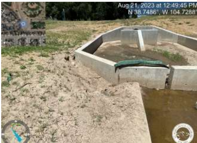
Photo 11: Pond: Fine grade rill erosion around the forebay and stabilize.
