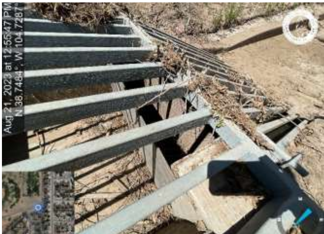
Photo 15: Pond: Install concrete cross-member or equivalent between the trash screen and orifice plate gap. Documents. Reference sheet C7.5 of the Construction Documents.
