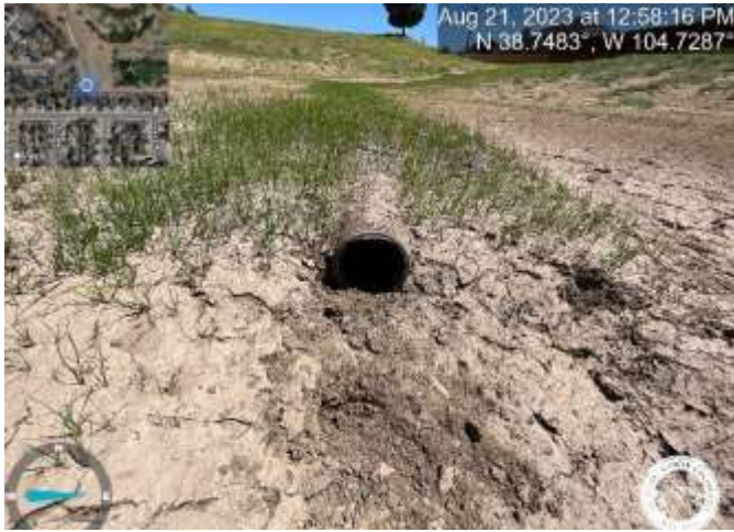
Photo 17: Pond: Show underdrain pipe on As-builts and update pond calculations as necessary if the underdrain generates more flow to the pond than previously
