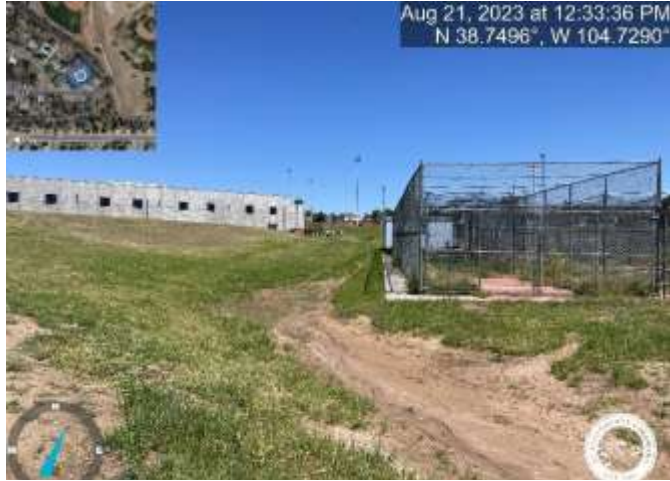
Photo 1: South of building: Install check dams within the drainage ditch per the approved plans. Reference sheet C8.2 of the Grading and Erosion Control Plans.
