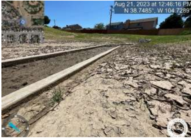
Photo 8: Raise pond bottom to top of trickle channel curb with a 3% slope towards trickle channel for positive drainage.
