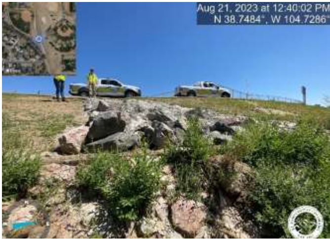
Photo 5: South of building: Remove and replace grouted riprap with 18" Type M riprap pad per the approved plans and for positive drainage and erosion prevention. The riprap needs to be shaped for positive drainage, currently the grouted riprap does not have a consistent shape with grouted rocks raised in the middle of the rundown. The riprap also should be buried in the ground so that the riprap is flush with the ground. Currently the riprap is a foot above the ground which is contributing to erosion from splashover especially downstream where the rundown meets the concrete lined channel. Reference sheet C8.2 of the Grading and Erosion Control Plans.
