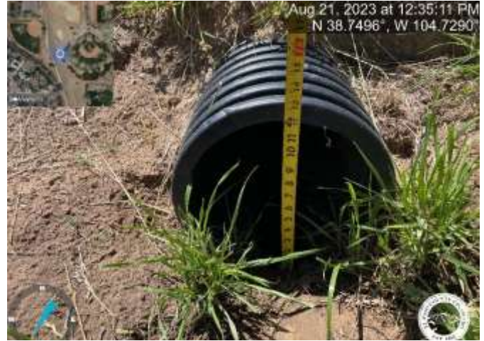
Photo 2: Above Grouted riprap: Replace 12" pipe with 24" RCP with a FES per the approved plans. Reference sheet C8.2 of the Grading and Erosion Control Plans.
