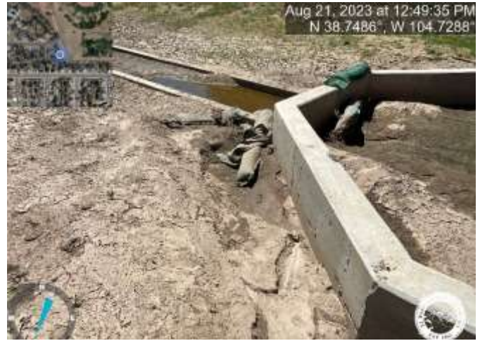
Photo 10: Pond: Fine grade rill erosion around the forebay and stabilize.
