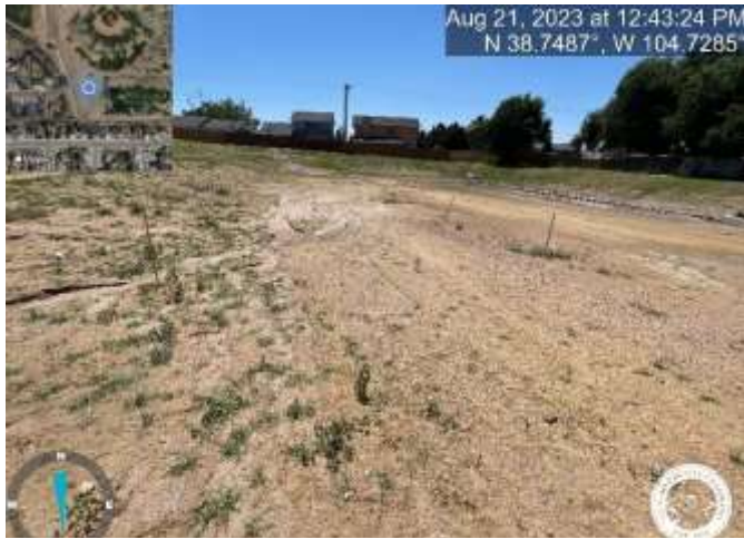
Photo 6: Pond: Remove excess sediment from the maintenance access road and reestablish road base.
