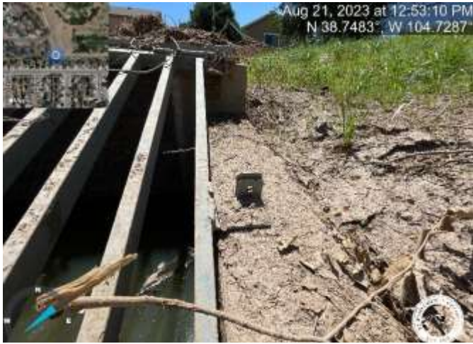
Photo 13: Pond: Install bolts or locks on grate per the approved plans. Reference sheet C7.5 of the Construction Documents.
