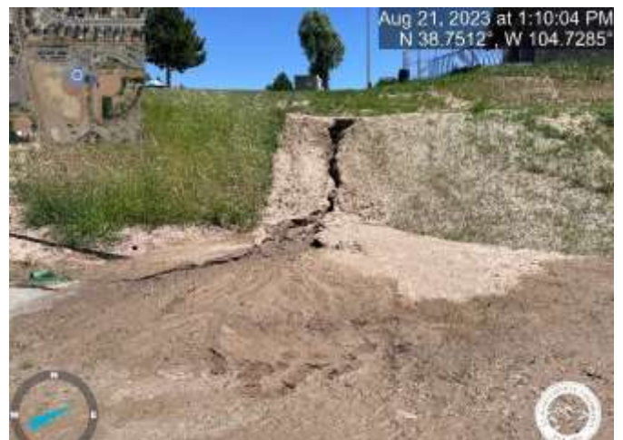
Photo 20: NE corner of the building: Repair blow out, fine grade, and stabilize slope.
