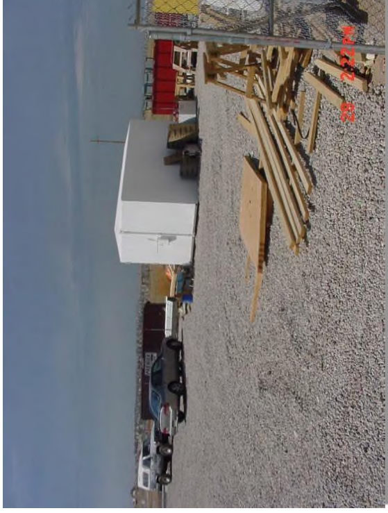
Photograph SSA-1. Example of a staging area with a gravel surface to prevent mud tracking and reduce runoff. Photo courtesy of Douglas County.
