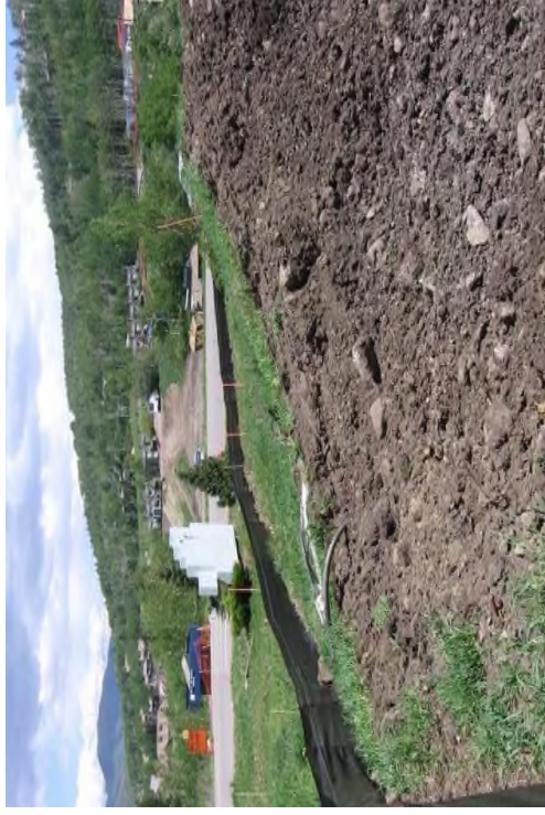
Photograph SP-1. A topsoil stockpile that has been partially revegetated and is protected by silt fence perimeter control.
