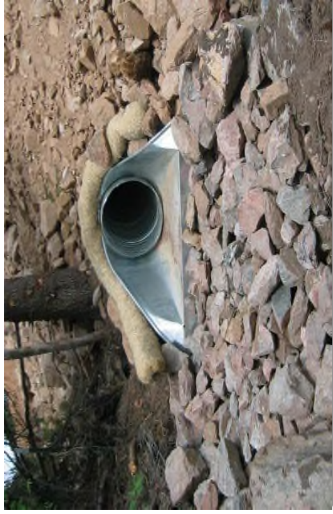
Photograph TOP-1. Riprap outlet protection.
