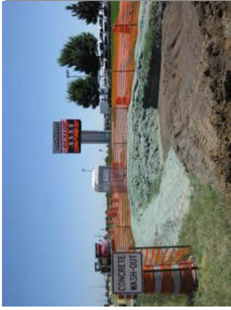
Photograph CWA-3. Earthen concrete washout. Photo courtesy of CDOT.
