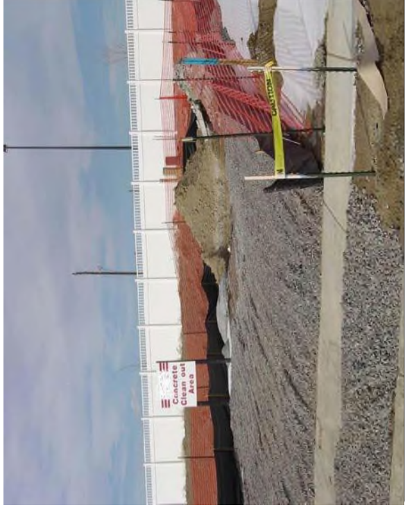
Photograph CWA-1. Example of concrete washout area. Note gravel tracking pad for access and sign.
