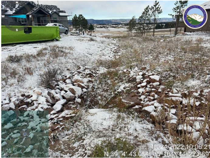
Photo 1: Add 12-inch rock as per plans along downgradient side of culvert D9b.
