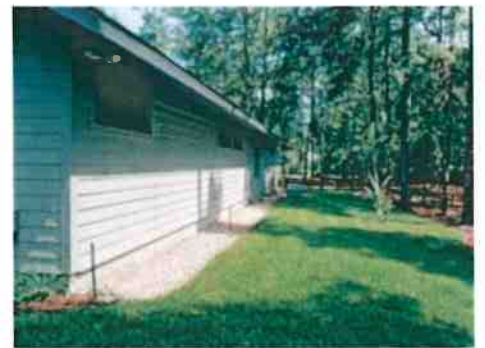
Use pebbles instead of mulch near the home's foundation where possible.
