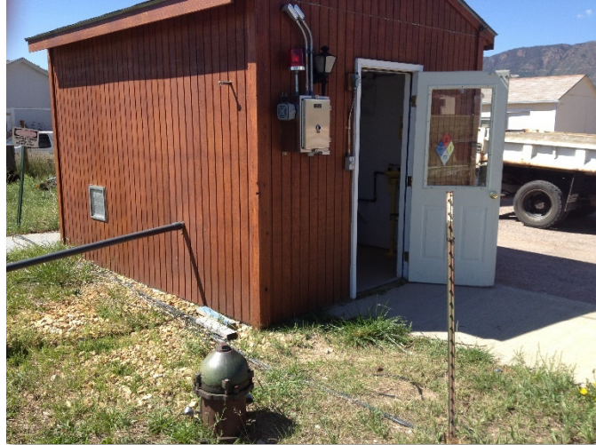
Figure 4-9: Well Head and Minor Treatment Facility
