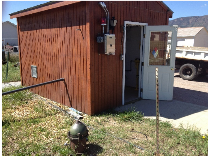
Figure 4-9: Well Head and Minor Treatment Facility
