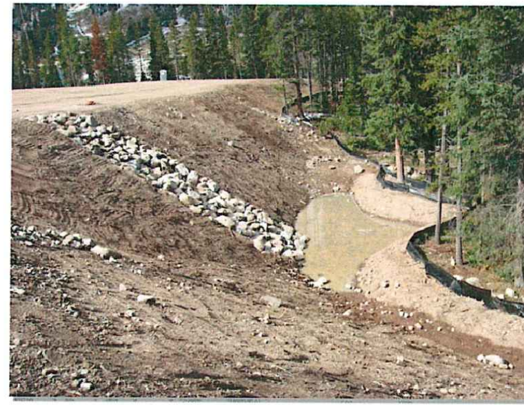
Photograph SB-1. Sediment basin at the toe of a slope. Photo courtesy of WWE.
