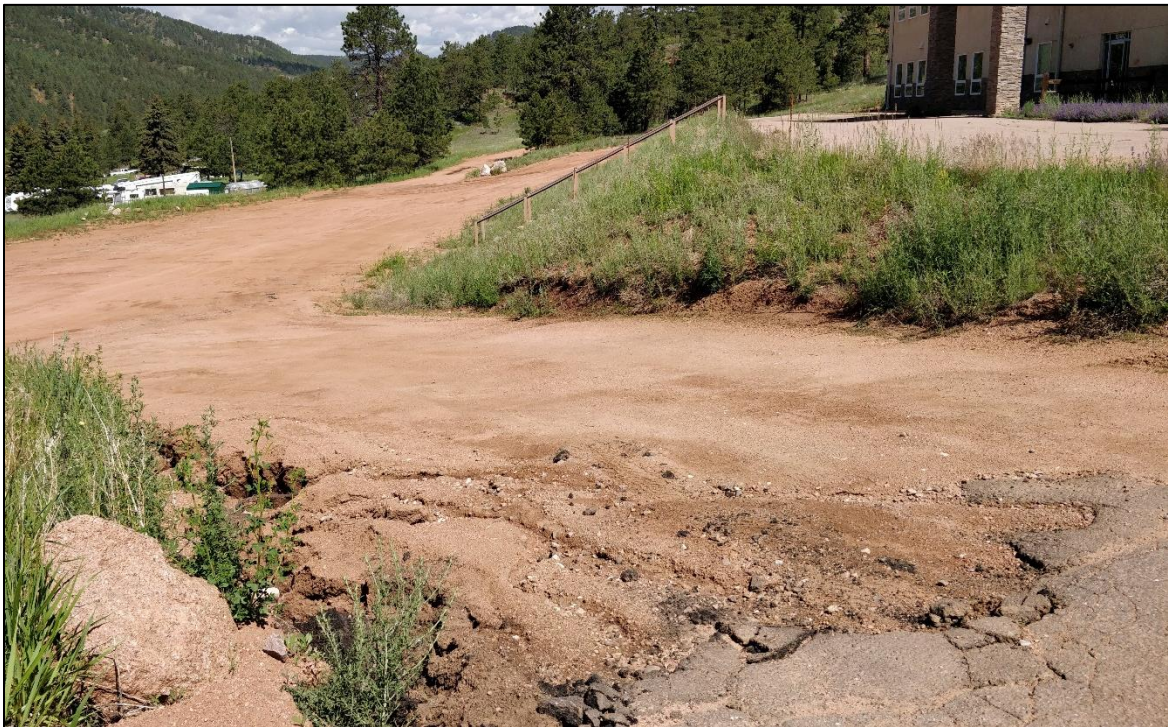
Photograph 2. Erosion of Existing Roadway Southeast of Building - Looking West
