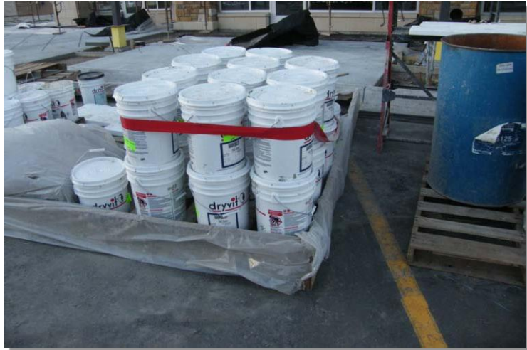
Photograph SPCC-1. Use of secondary containment around supplies stored outside helps to reduce the likelihood of spill and leaks reaching the storm sewer system in runoff. Photo courtesy of Tom Gore.
