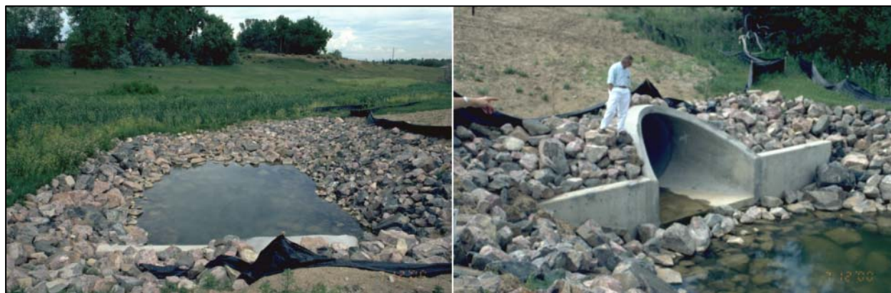
Photograph HS-12—Upstream and downstream views of a low tailwater basin in Douglas County protecting downstream wetland area. Burying and revegetation of the rock would blend the structure better with the adjacent terrain.
