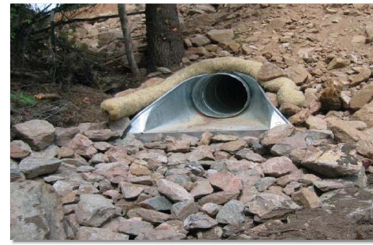
Photograph TOP-1. Riprap outlet protection.
