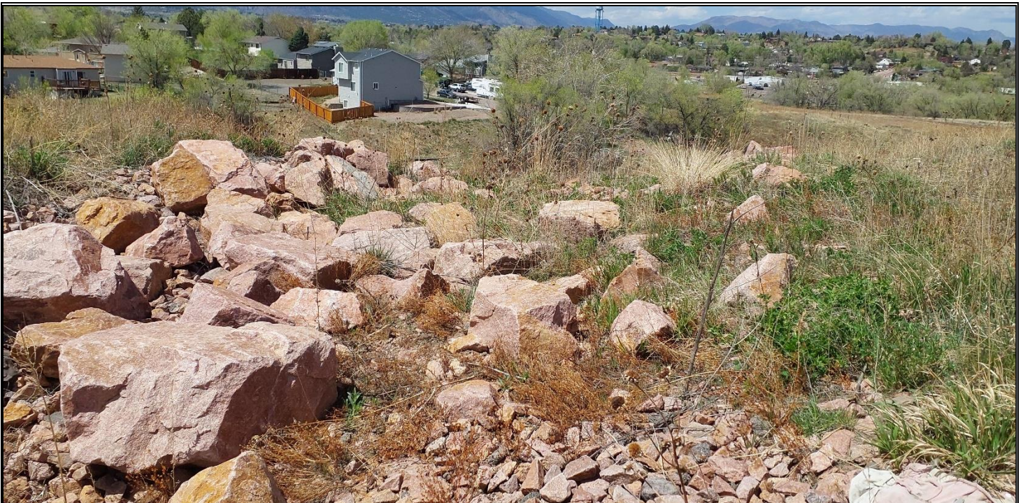
Photo No: 10 Direction Photo Taken: Northwest Figure No: 4 Description: A cobble riprap line drainage swale located at the northwestern portion of the sediment basin.
