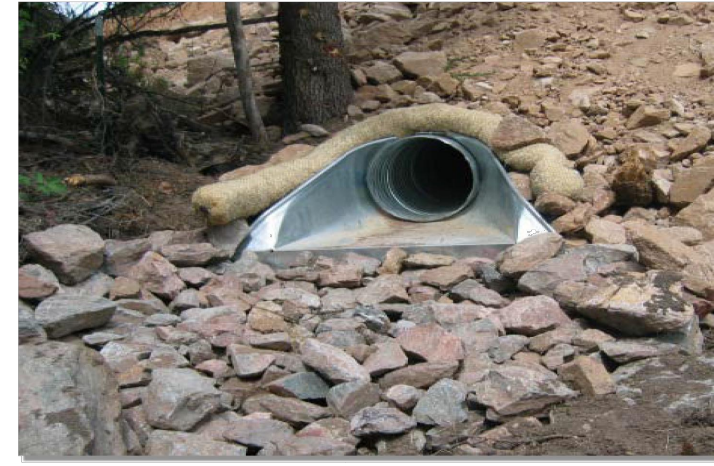
Photograph TOP-1. Riprap outlet protection.
