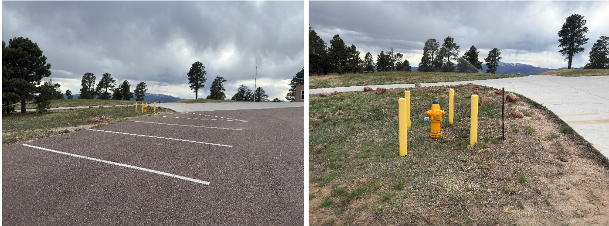
Figure 1: Existing Fire Hydrant at Clubhouse
