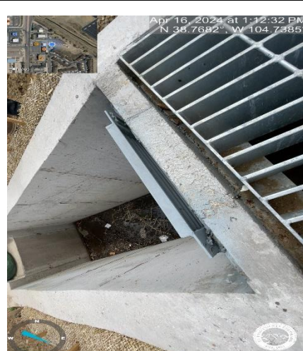
Photo 2: Pond: Alleviate gap between the trash rack and concrete structure.
