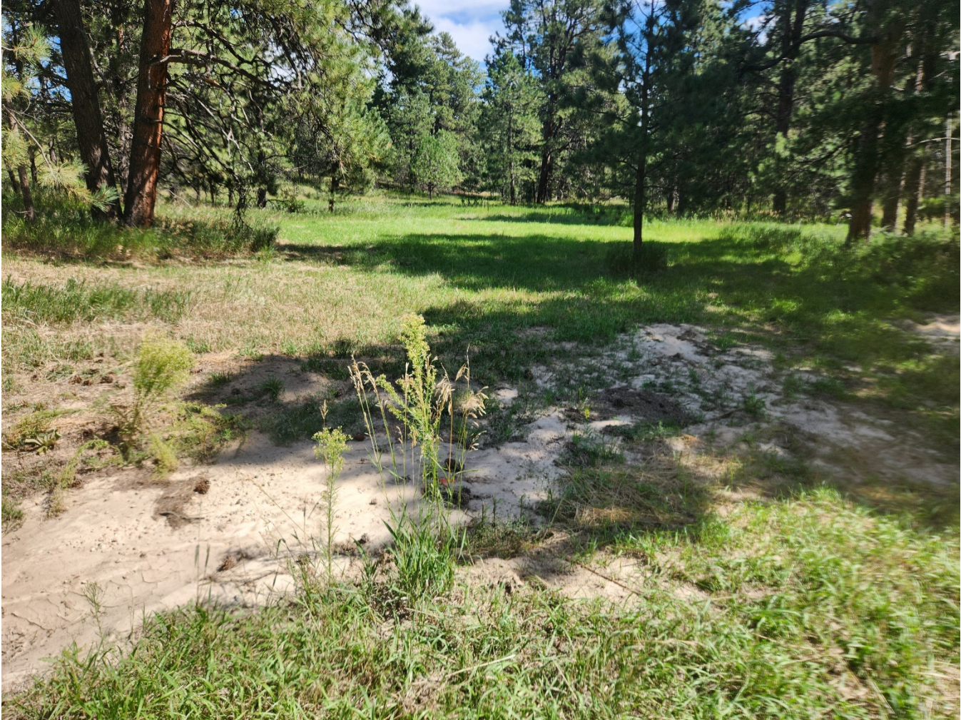
Figure 9: Double 12" PVC culverts, tailwater channel
