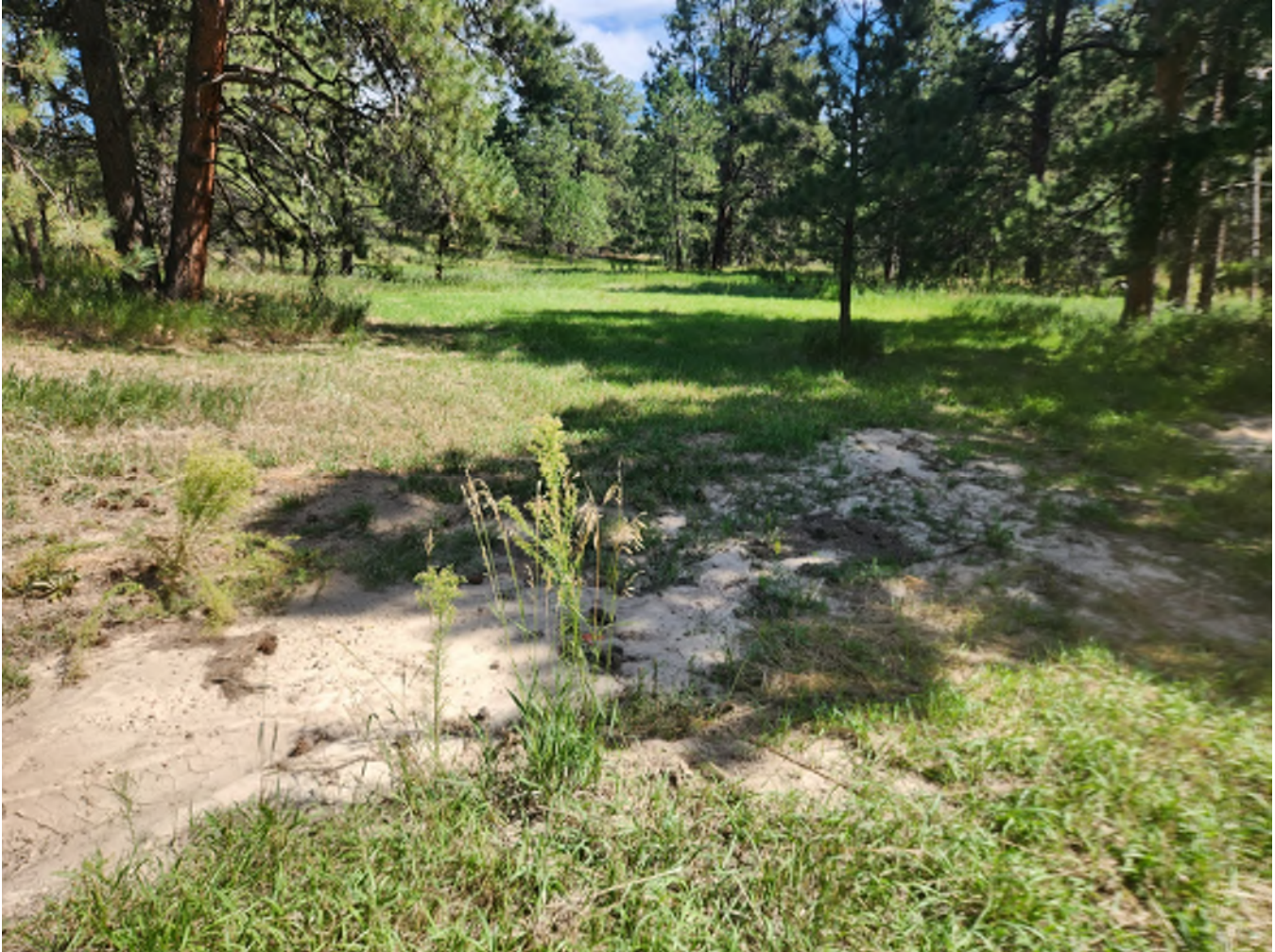
Figure 9: Double 12" PVC culverts, tailwater channel
