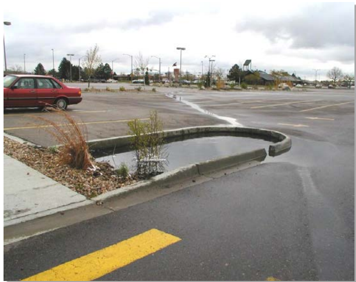
Photograph B-4. Runoff passed the upgradient rain garden, shown in Photo B-3, and flooded this downstream rain garden.
