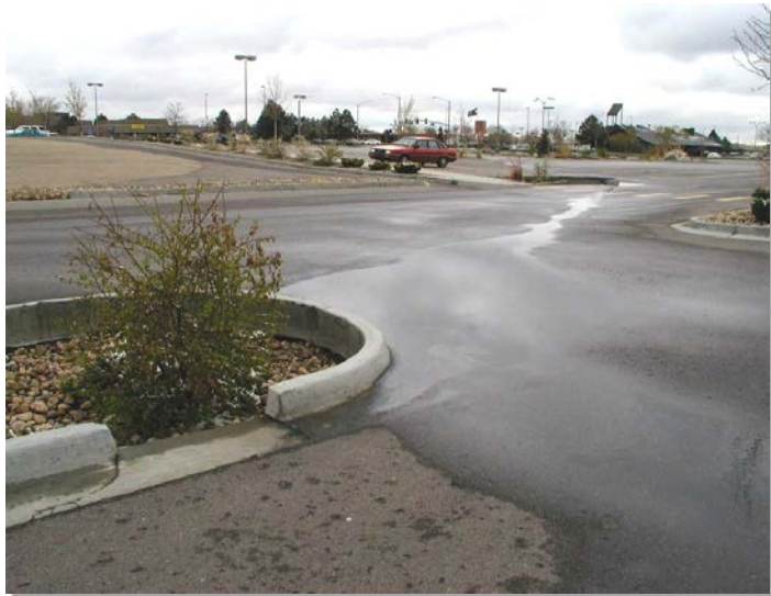
Photograph B-3. Inadequate construction staking may have contributed to flows bypassing this rain garden.
