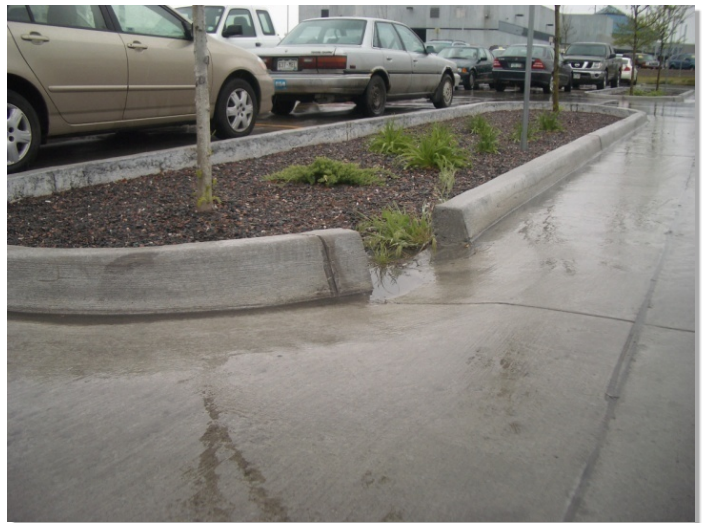
Photograph B-4. The curb cut shown allows flows to enter this rain garden while excess flows bypass the facility.
