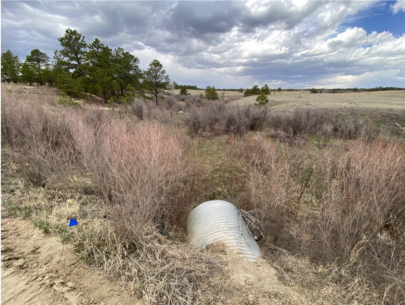
Another view of the wetlands north of Arroya Lane as seen from the roadway, facing north. The pines of the Black Forest can be seen in the distance, with a few creeping down the slopes toward Sand Creek. The large culvert conveys flows under the road.
