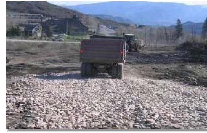
Photograph VTC-1. A vehicle tracking control pad constructed with properly sized rock reduces off-site sediment tracking.
