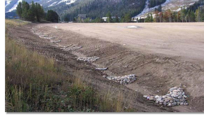
Photograph CD-1. Rock check dams in a roadside ditch. Photo courtesy of WVE.
