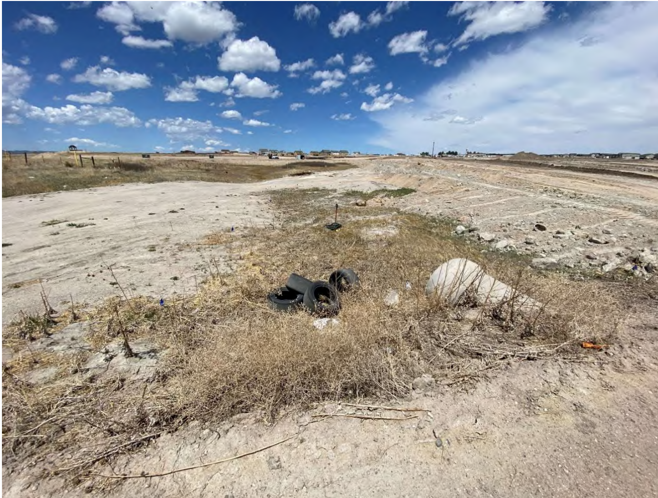
W4 and W5 – North-facing view from the construction road crossing south of W4. Darker brown areas are areas where wetland vegetation can be found, surrounded by areas impacted by grading. The culvert that connecting W4 to W6 is seen on the right side. Grading for Sterling Ranch Road can just be seen as a raised road grade just beyond W5 in the distance.
