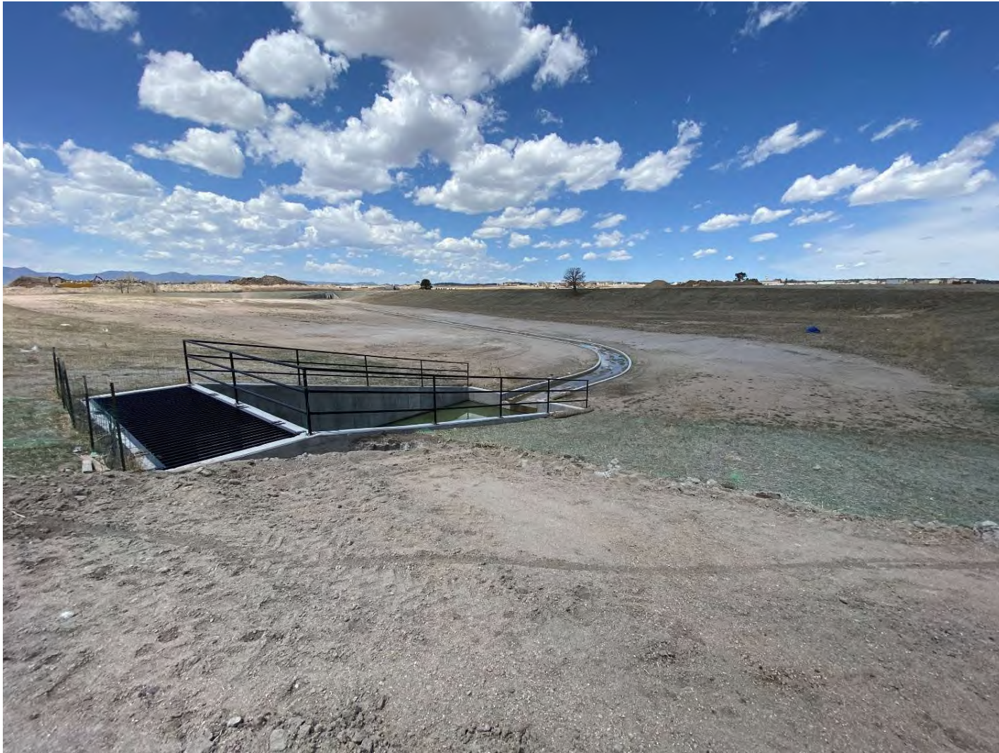
View of the detention basin located south of W6, facing NW. Stormwater flows from the surrounding development are piped into this basin, which lacks surface connection to any of the wetlands on the Project site.
