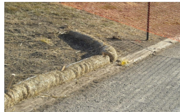
Photographs SCL-1 and SCL-2. Sediment control logs used as 1) a perimeter control around a soil stockpile; and, 2) as a "fishhook" perimeter control at the corner of a construction site.
