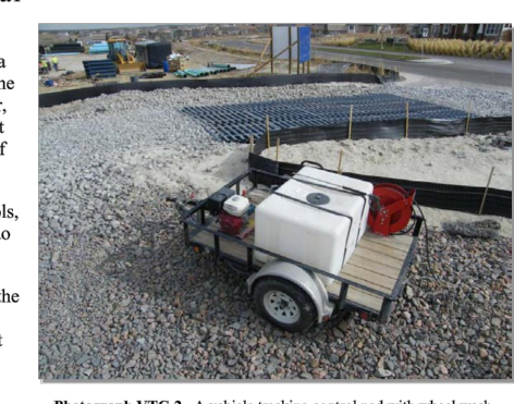
Photograph VTC-2: A vehicle tracking control mat with wheel wash facility. Photo courtesy of Tom Coen.
