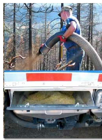
Photograph CB-1. Application of a compost blanket to a disturbed area. Photo courtesy of Caltrans.
