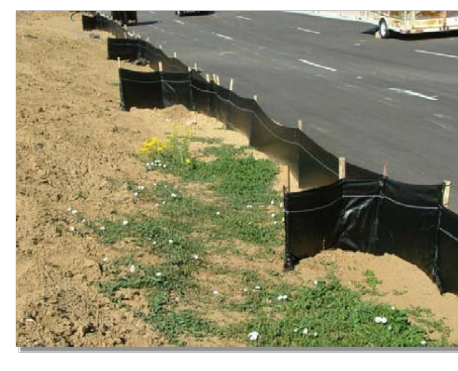
Photograph SF-2. When silt fence is not installed along the contour, a "J-hook" installation may be appropriate to ensure that the BMP does not create concentrated flow parallel to the silt fence. Photo courtesy of Tom Gore.
