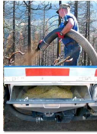
Photograph CB-1. Application of a compost blanket to a disturbed area. Photo courtesy of Cattaraugus.
