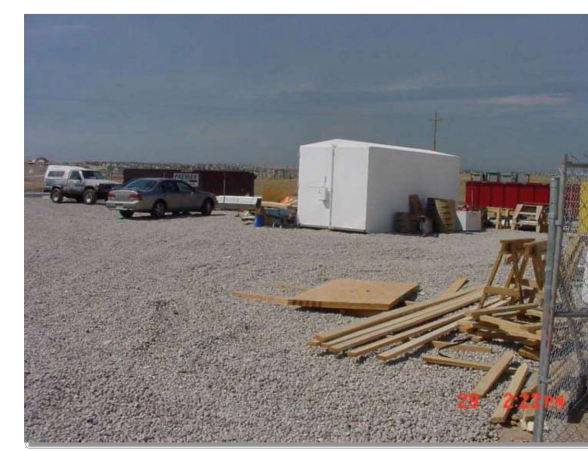
Photograph SSA-1. Example of a staging area with a gravel surface to prevent mud tracking and reduce runoff.
