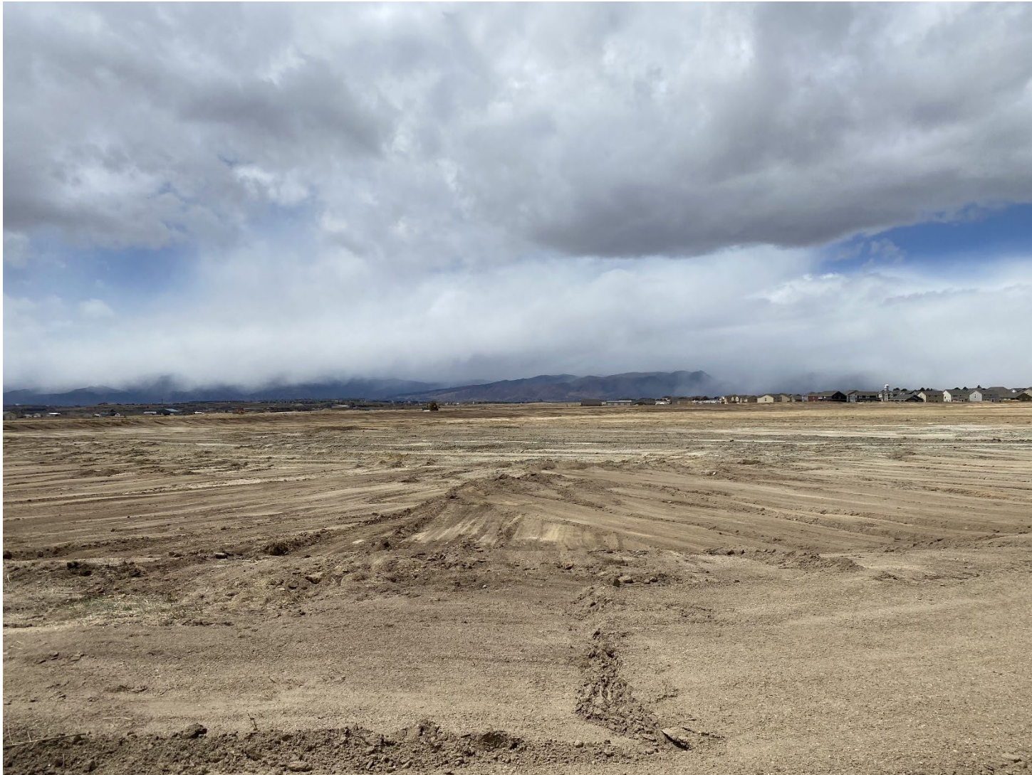
PHOTO 2 – View of the disturbed areas of the site near the south-central portion, facing southwest. Flora and fauna are nonexistent in these areas, and earth-moving activities are ongoing.
