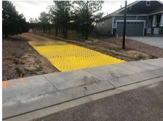
VTC installed at Willow Park Drive as per CE1.1.
