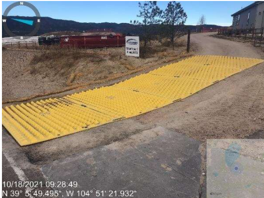
VTC installed as per plans off of Lake Woodmoor Drive.
