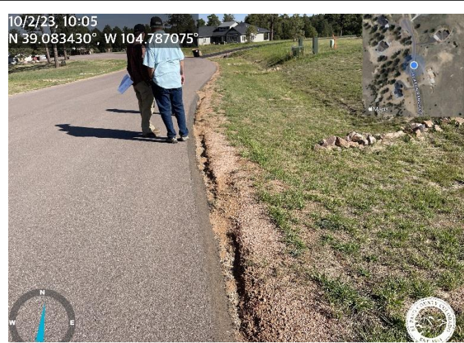
Photo 1: Regrade Jackson Ranch Ct shoulder per detail on each side of the road.
