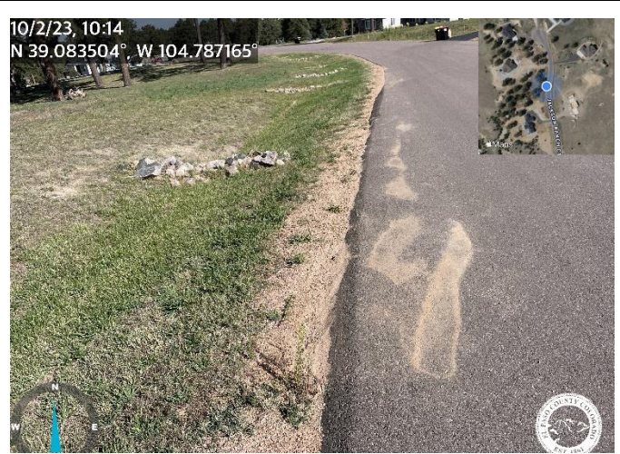
Photo 2: Regrade Jackson Ranch Ct shoulder per detail on each side of the road.
