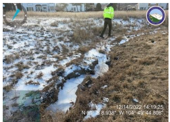
Photo 2: Address severe erosion in Swale K.
