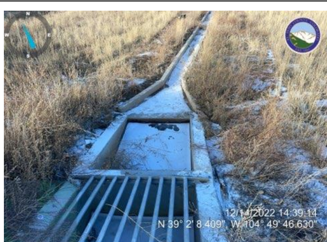
Photo 4: Where trickle channel meets micropool is not installed per approved plans; corners do not tie into the walls in the field.
