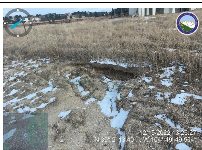
Photo 5: Repair erosion along concrete swale behind Lots 6-8 west of Stone Eagle Place.
