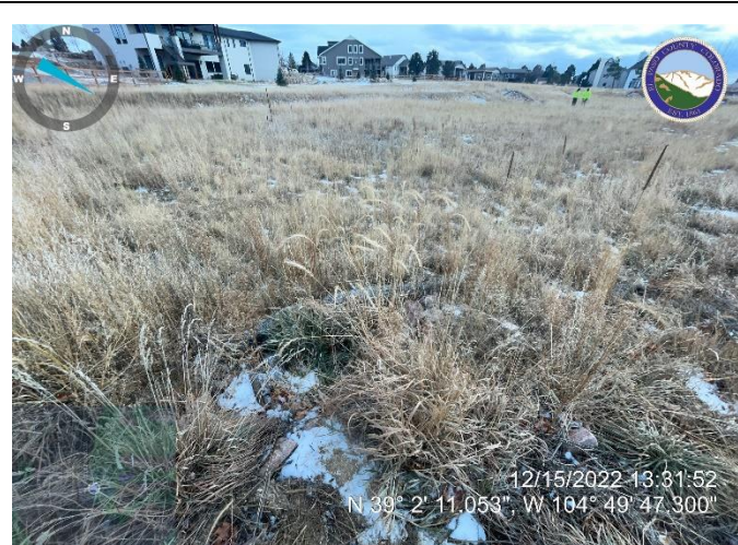
Photo 3: Remove straw wattle temporary control measure from upstream side of Swale J.
