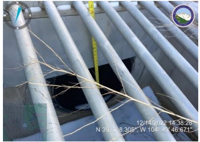
Photo 8: Restrictor plate not installed at correct height
