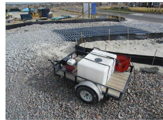
Photograph VTC-2. A vehicle tracking control pad with wheel wash facility. Photo courtesy of Tom Gore.
