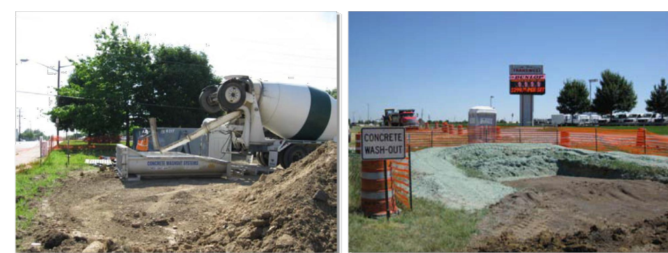
Photograph CWA-2. Prefabricated concrete washout. Photo courtesy of CDOT. Photograph CWA-3. Earthen concrete washout. Photo courtesy of CDOT.
