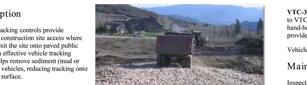
Photograph VTC-1. A vehicle tracking control pad constructed with properly sized rock reduces off-site sediment tracking.
