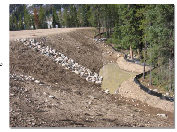
Photograph SB-1. Sediment basin at the toe of a slope. Photo courtesy of W.W.
