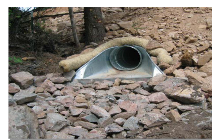
Photograph TOP-1. Riprap outlet protection.
