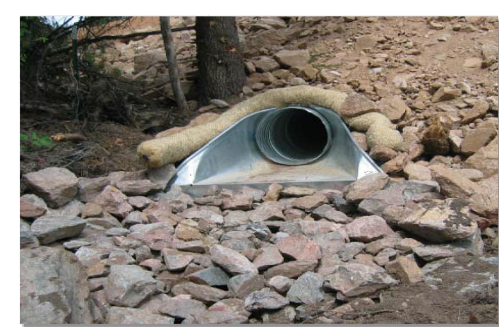
Photograph TOP-1. Riprap outlet protection.
