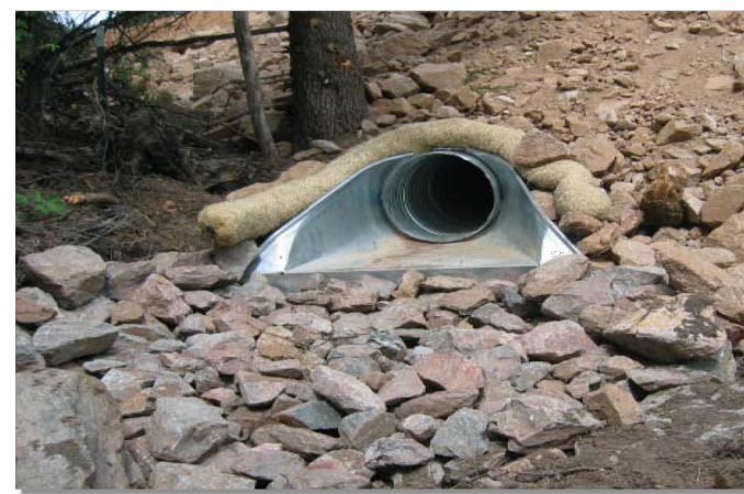
Photograph TOP-1. Riprap outlet protection.
