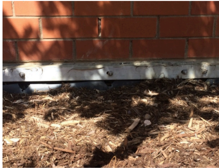
Photograph B-2. The impermeable membrane in this photo has ripped from the bolts due to placement of the media without enough slack in the membrane.
