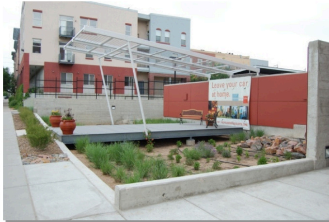
Photograph B-1. This recently constructed rain garden provides bioretention of pollutants, as well as an attractive amenity for a residential building. Treatment should improve as vegetation matures.
