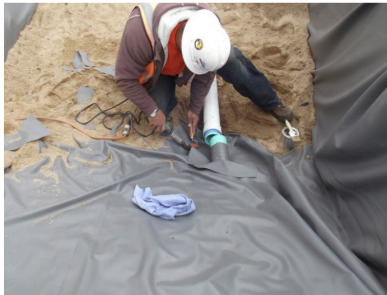
Photograph B-3. Ensure a water-tight connection where the underdrain penetrated the liner. The heat-welded “boot” shown here is an alternative to the clamped detail shown in Figure B-2.
