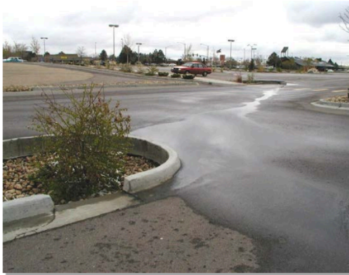
Photograph B-3. Inadequate construction staking may have contributed to flows bypassing this rain garden.
